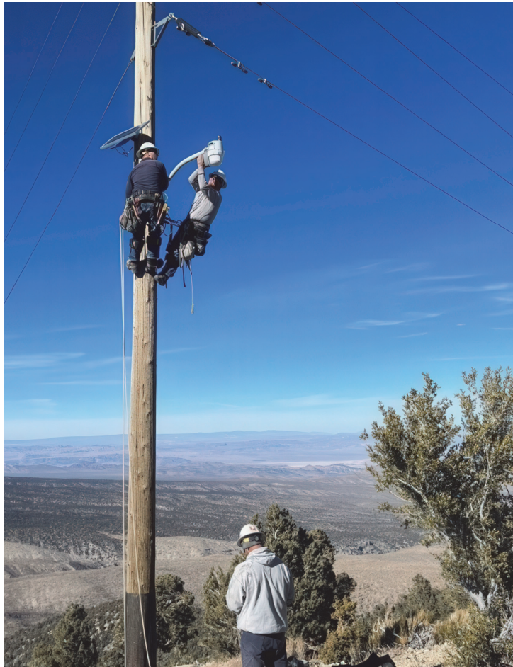
Installation of a FIREBird device in a Wildland-Urban Interface community
